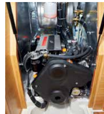
Room around the engine can be increased by removing panels in the aft cabin, making access very good
